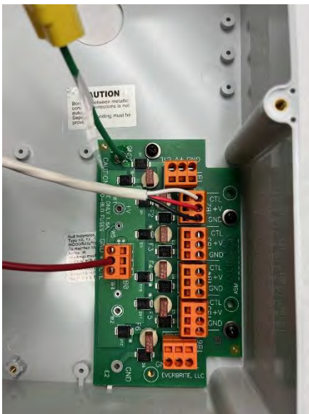
Figure 11: Fuse Box Wiring
