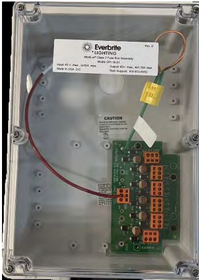
Figure 6: Distribution Panel / Fuse Box
